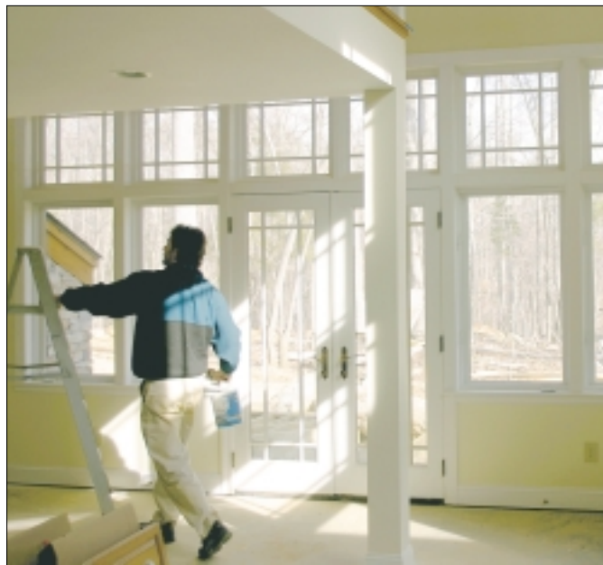
Painter David Spencer works in a home being constructed in North Durham County by Seteve Brouillard's crew of craftsmen and designed by architect Barry Swanson, AIA.
