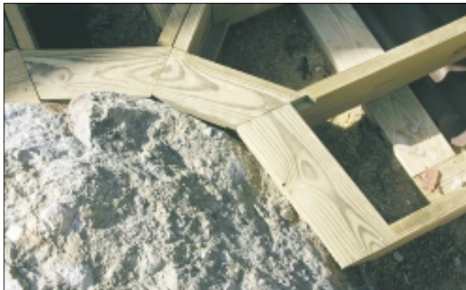
The deck frame at the Brouillard site has been crafted to fit around several large rock formations.
